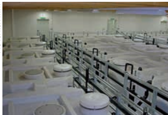
PVS VOPROM WWTP
