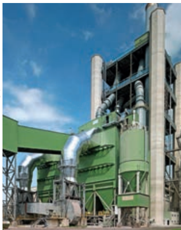
Dedusting plant for Cement Mill
